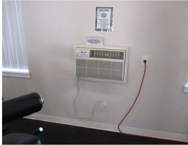
This is the wall mounted Frigidaire Air Conditioner located in the fitness center.
