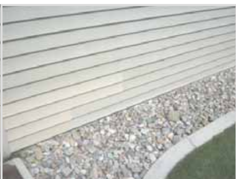
An example of limited repairs which gives a "patched" appearance to the building.
