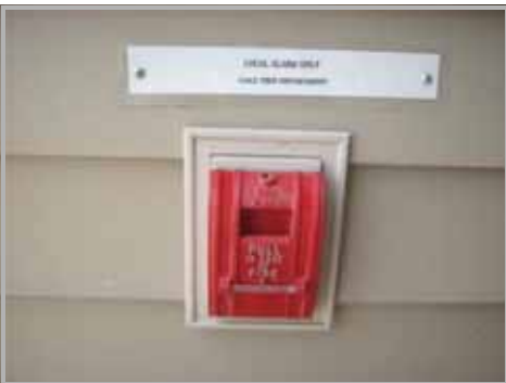
Pull stations are located in the breezeways of the each three story buildings.
