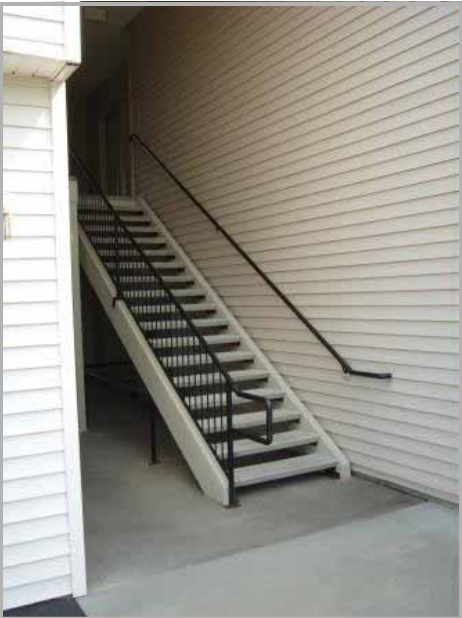
Periodic repairs to concrete walks and the concrete stair treads will be required in the future.
