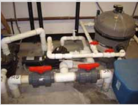
The pool pumps, filters, motor and heater are all well maintained throughout both the Winter and Summer months
